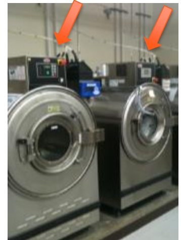
Ozone Injection Tubing
